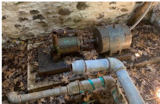
Pump (center rear), Motor (right rear), w/ pipes foreground
